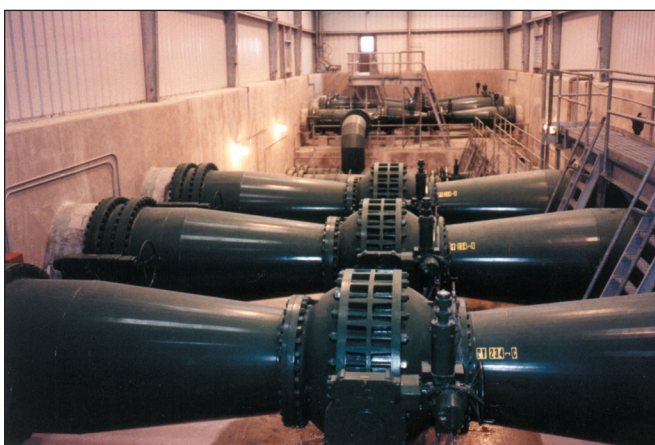
Ball valve in distribution pump station.
